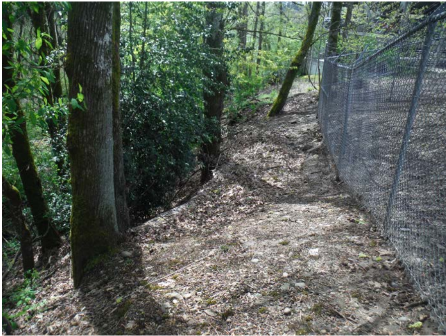
Photo 9: 90 th Pump Station, potential slide along the western limit of the site, looking south, (April 9, 2018).
